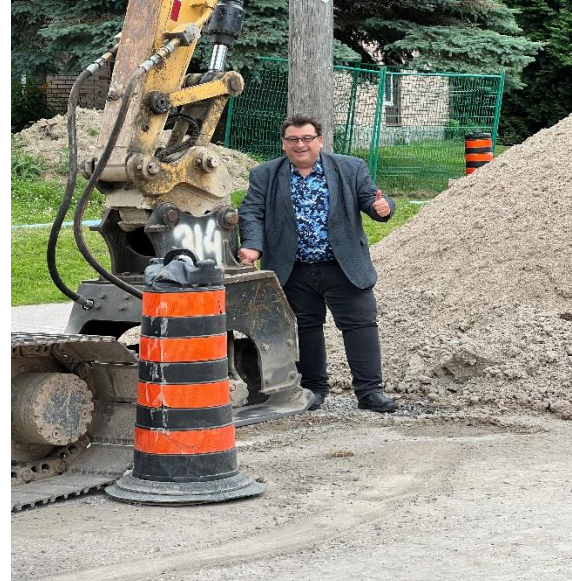
Councillor Peter Dykie at the Agar Avenue/Davey Boulevard/Miller Park Avenue project site.
