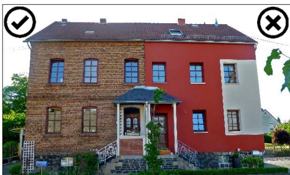
An extreme example of over cladding where the right side of the brick masonry façade is covered with EIFS (Source: Handwerker)
