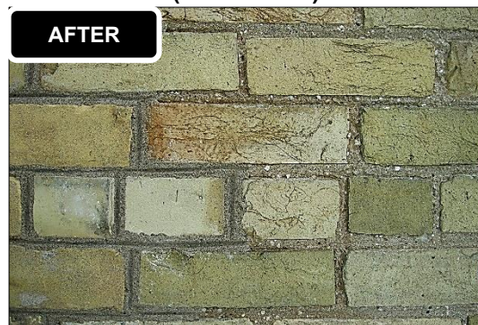
New lime rich mortar is applied to the joints. Repointing work is complete. (Source: GDV)
