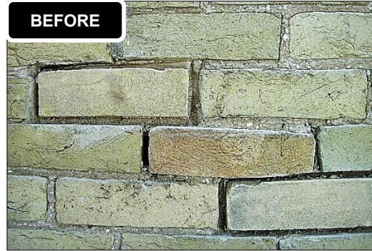
Deteriorated mortar joints require repointing. Deteriorated joints are cut-out using handheld tools prior to repointing. (Source: GDV)
