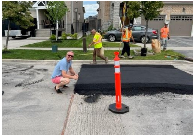
15: Councillor Joseph Giordano at project site where contractors are installing a speed bump on the roadway
